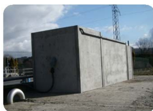
Planta experimental instalada
