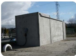
Planta experimental instalada
